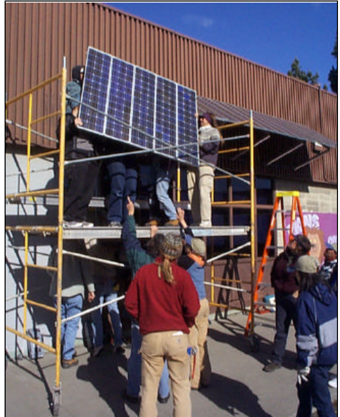
Fig. 5 Women from a Solar Energy International solar installation workshop hoist solar panels at Lincoln Middle School in Alameda. Not only will the solar system have a lasting impact, but the process in which it was installed, provided an educational experience.
