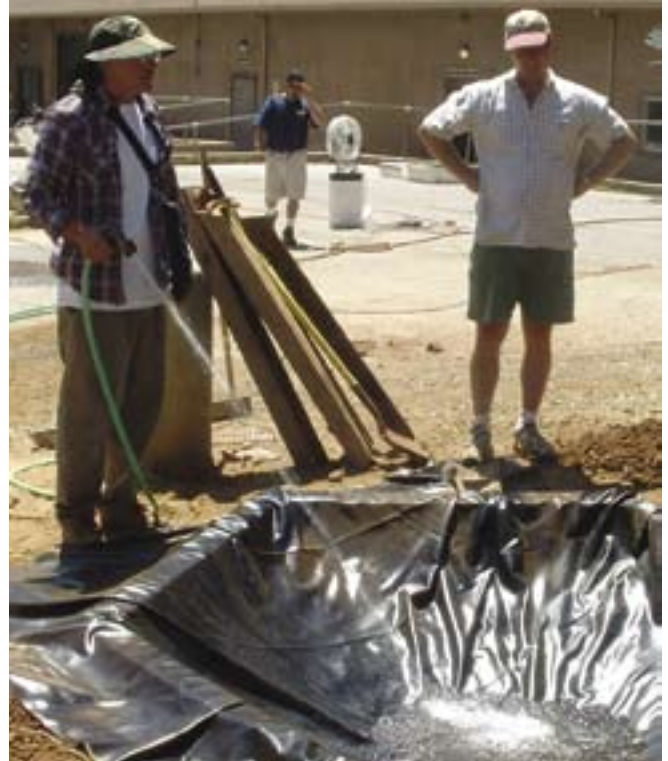
The liner is laid into the hole dug for the fountain basin and across the fountain curb. Water is added before the liner is tacked to the wooden curb to allow for an unstressed fitting.
