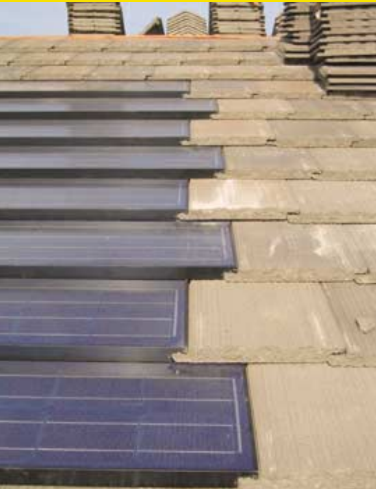
Solar Panels seamlessly integrated with a concrete tile roof.
