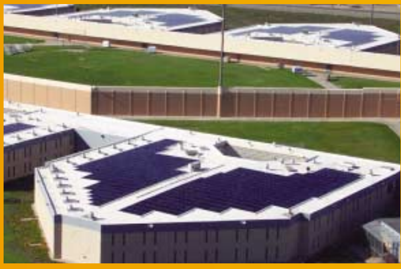
At the Santa Rita jail in Dublin, California, solar panels work together with a reflective roofing material to keep the inside of the facility cooler.
